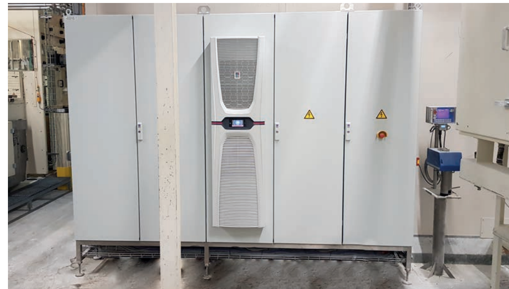
Zum FAT (Factory Acceptance Test) werden alle Retrofit-Komponenten bei WDS in Betrieb genommen. For the FAT (Factory Acceptance Test), all retrofit components are put into operation at WDS.
